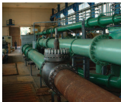
Figure 2: Swing check valve with disk position fixation in the test rig
