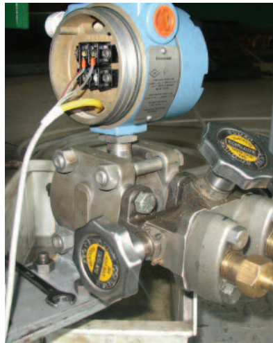
Figure 5: Differential pressure gauge Rosemount with connecting valves
